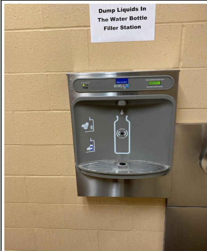
2/7/2024 - 1204-9 - Intermediate School - Outside Girls Restroom - Left
