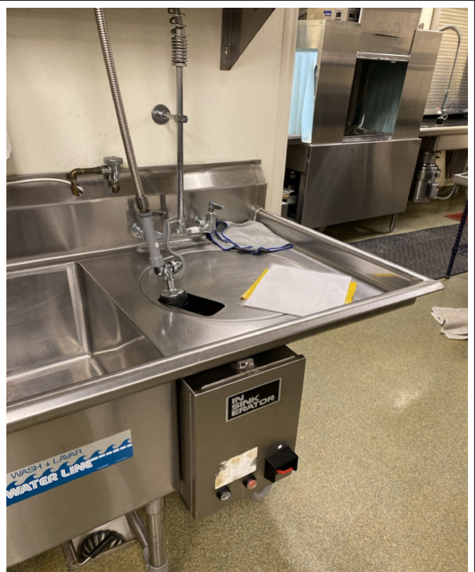
2/7/2024 - 1204-16 - Intermediate School - Kitchen - Three Bay Sink-Right
