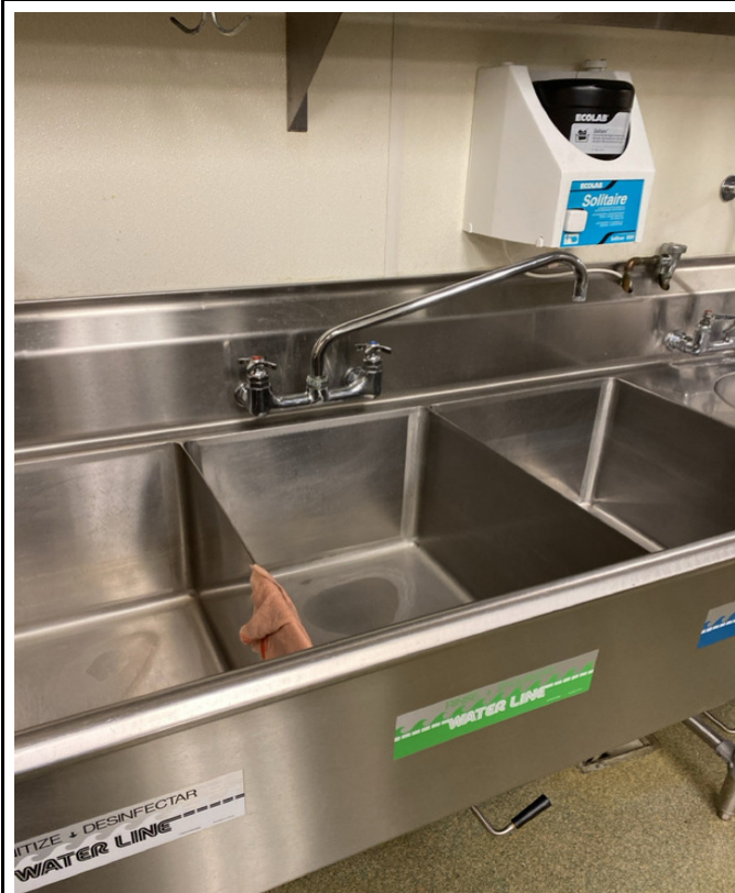
2/7/2024 - 1204-15 - Intermediate School - Kitchen - Three Bay Sink - Left
