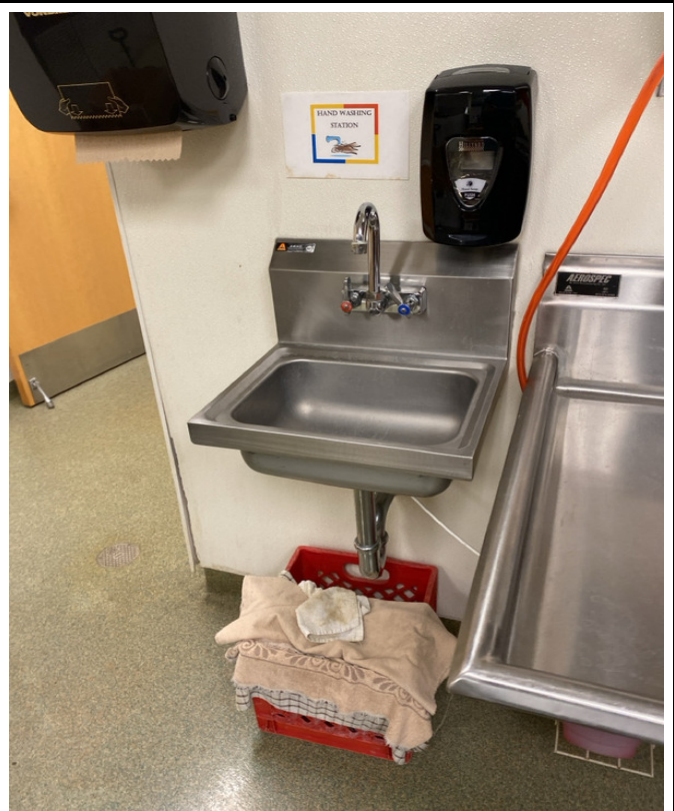
2/7/2024 - 1204-14 - Intermediate School - Kitchen - North Handwashing Sink
